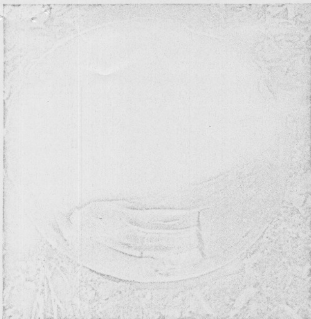
FIGURE 4.—BITUMINOUS-COATED ASBESTOS-BONDED PIPE SHOWING SEVERE CRACKING OF PAVEMENT AT OUTLET END.
