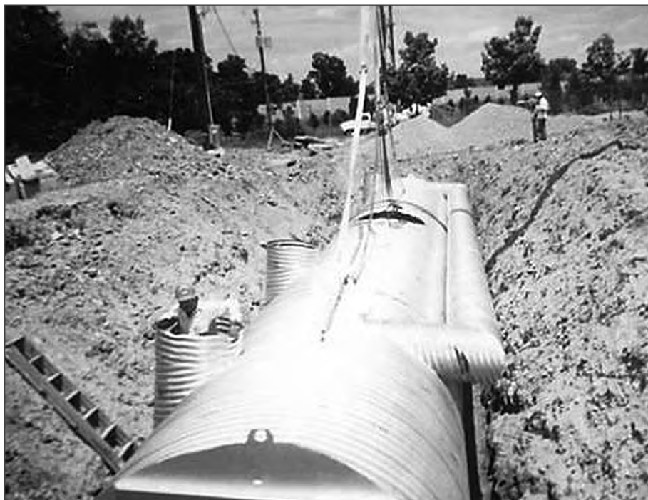
■ CSP sand filter system
