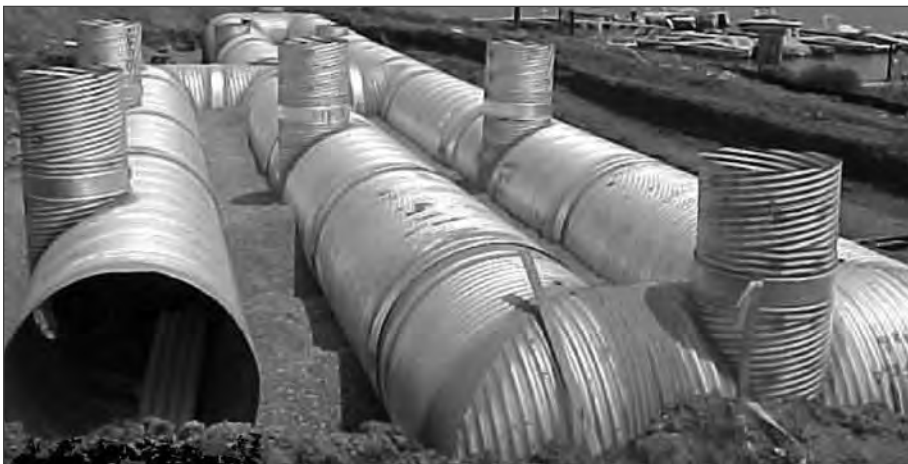
■ CSP riser manholes in underground detention system.
