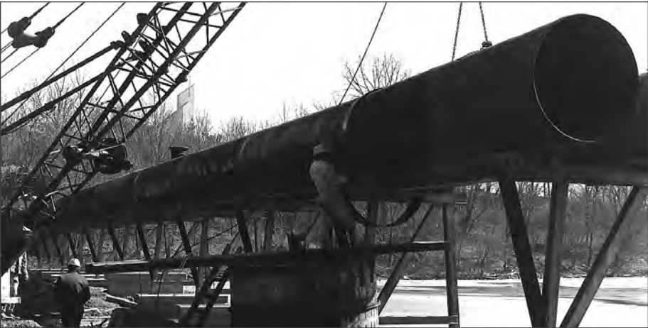
■ Corrugated steel pipe aerial sewer.
