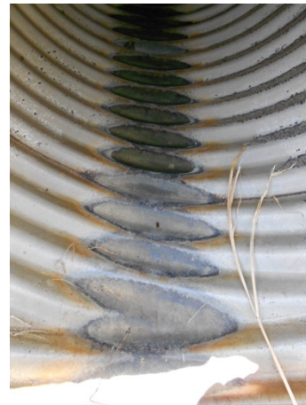
Figure 10. Coating removed due to bed load
