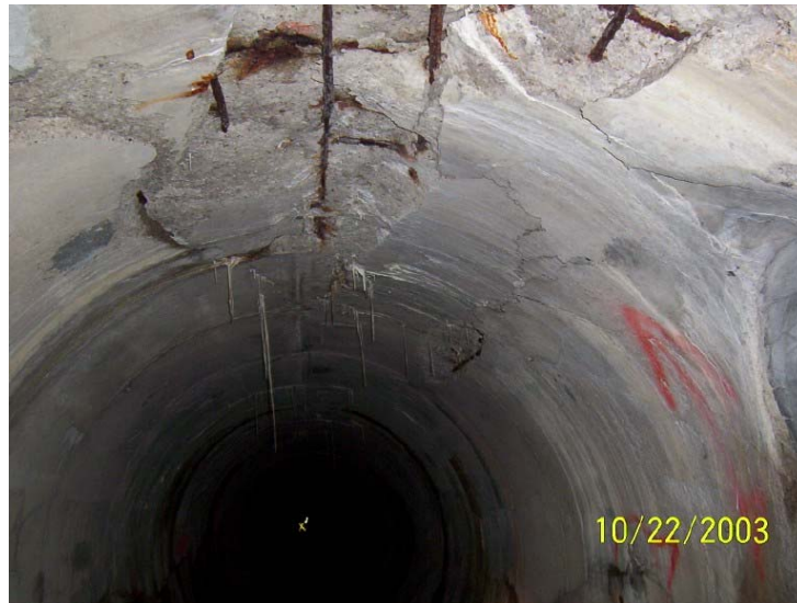
Cracked and Corroded Rigid Sewer Pipe
